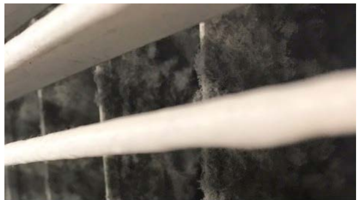
Excessive mold spores growing out of an air duct that has not been cleaned in years. (Photo by Clean Kenwood Coalition)
