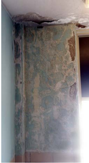
Chicago Academy High School. Severe water damage to interior wall, likely due to numerous cracks in the foundation and masonry or the leaky roof as noted in the 2014-2015 facility assessment . (Photo by Jim Cavallero)
