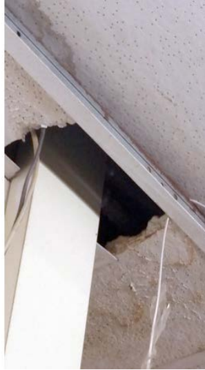
Kenwood High School. Asbestos ceiling tiles in physical education office that has become severely damaged and friable due to a boiler leak a few floors above. This led to dust covering the desks of some Kenwood teachers, including one who was pregnant at the time. (Photo by Sarah Rothschild)
